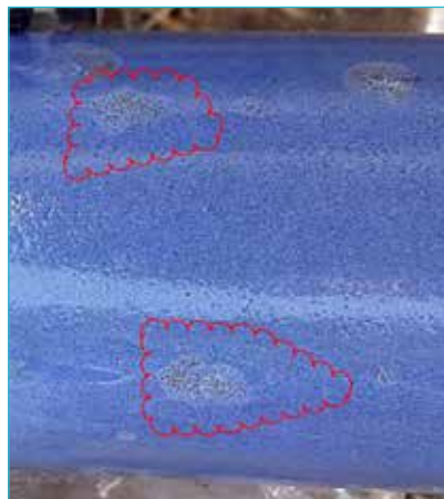
Figure 26: Crack or spalling on ceramic coating
