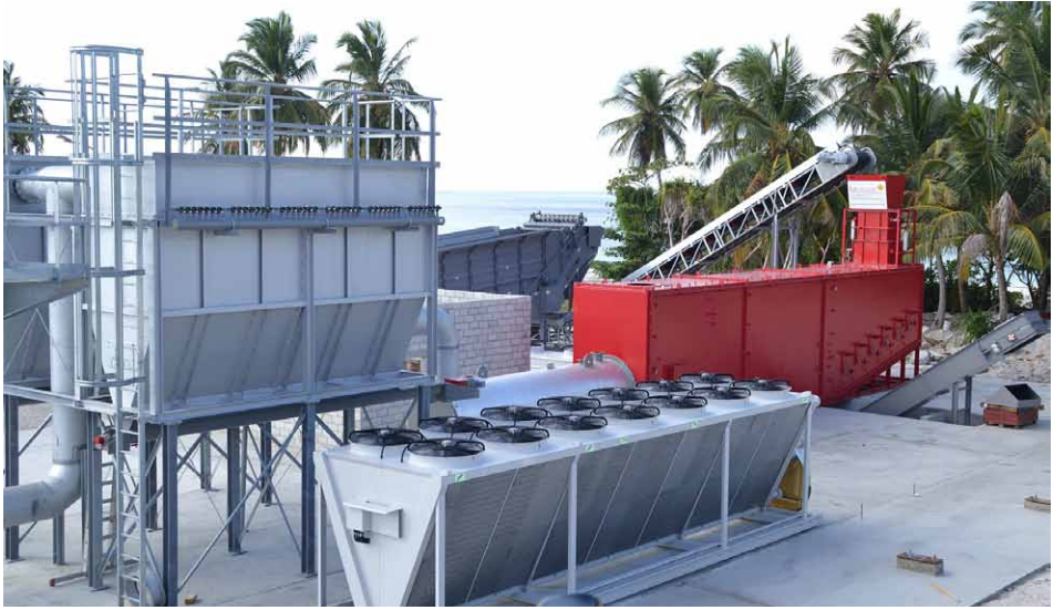
Figure 6: View to the incinerator, back house filter and air cooler
