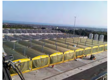
Figure 16: Biological Treatment GORE Cover showing 45 out of 60 modules during construction; Handling Cover: Hydraulic frame
